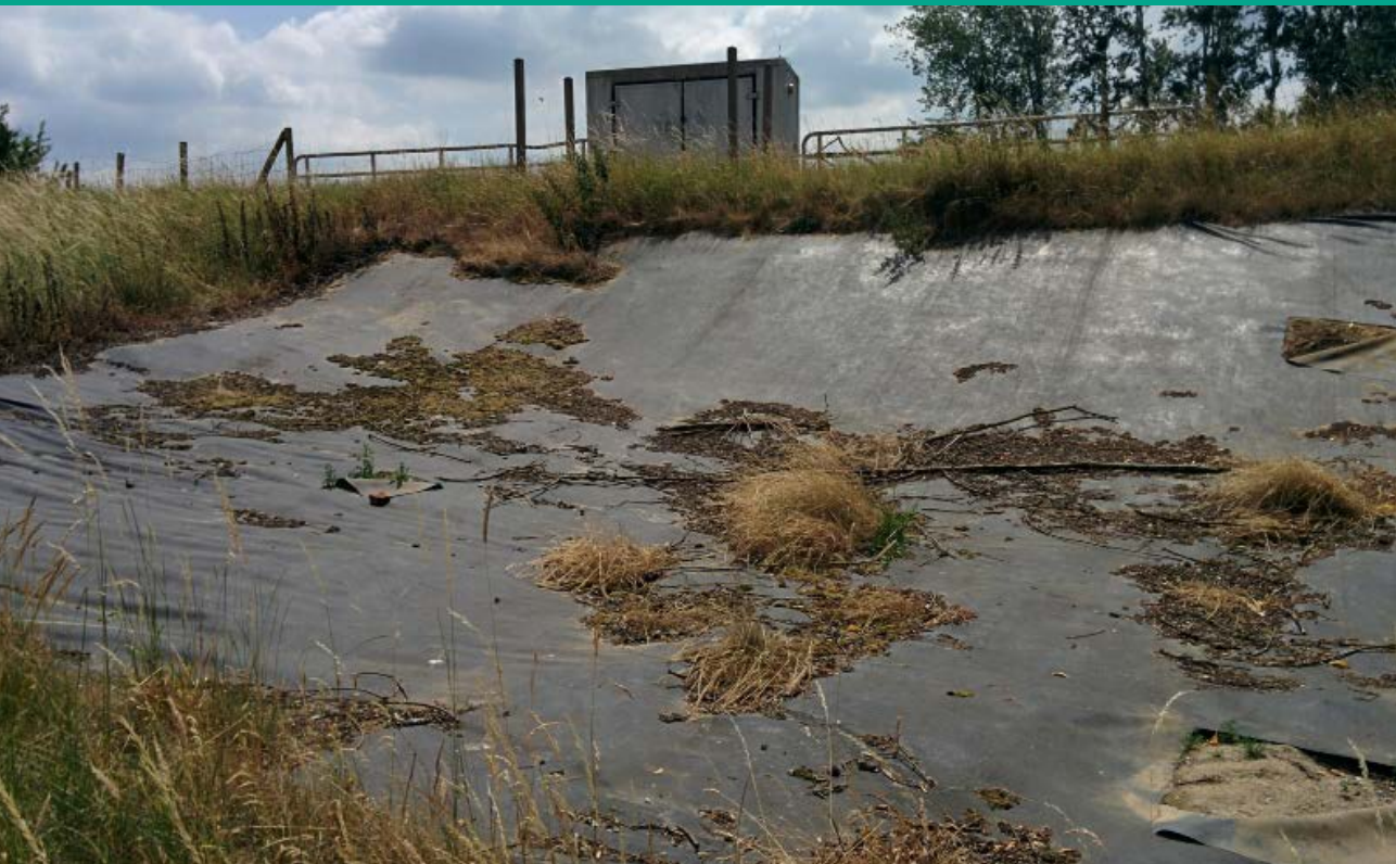
Fig 3. It is necessary to check for any damages that would allow the plant to grow through the sheeting. Photo: Marijke Thoonen
